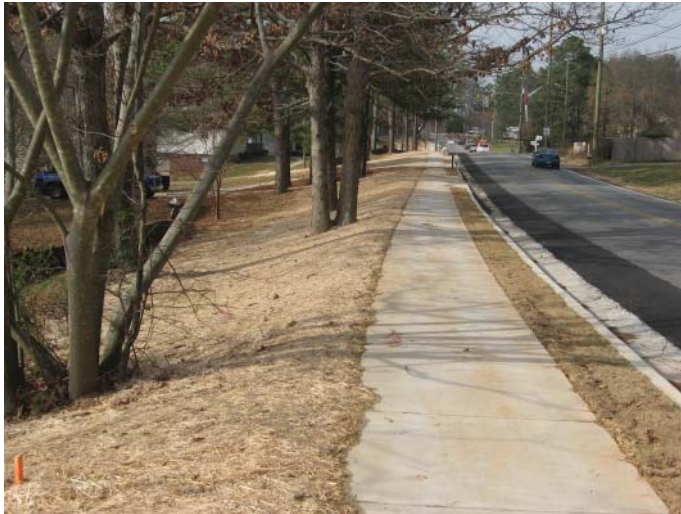
Figure 8. Trees disturbed by road and sidewalk construction
