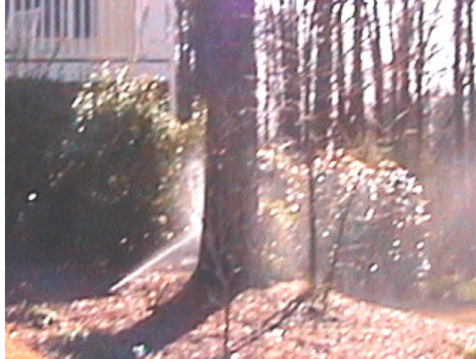
Figure 4-3. Poor design and/or installation of the applicator location wastes water because the sprinkler pattern is blocked by a tree 35 inches from the applicator.
